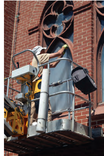
The recent St. Mary's restoration project also included a tedious restoration of re-leading and repairing a number of the stained glass windows in the church, a process that involved cleaning the glass, replacing the deteriorated lead between the glass panels, and repairing and painting the decorative wood surrounding the window.
